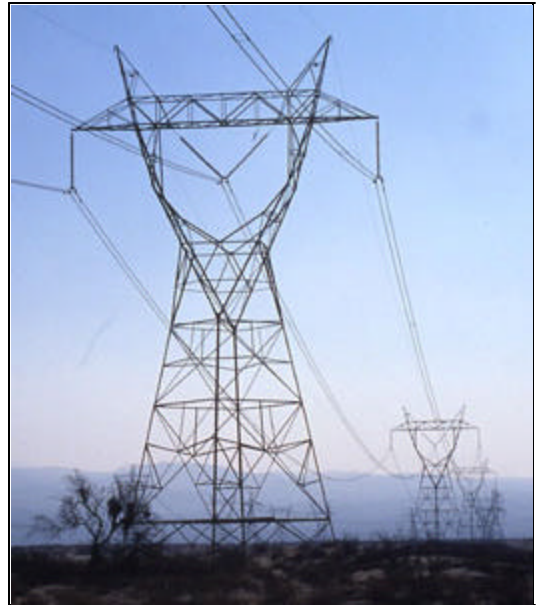
High-voltage transmission towers march across Southern California. The state is considering a process for designating transmission corridors. Photo by Sean Ramsay. Courtesy of The Energy Overseer.
